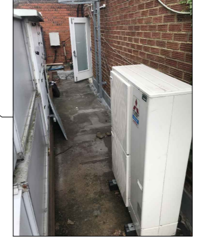
MITSUBISHI ?? CONDENSING UNIT ANTICIPATED SOUND PRESSURE LEVEL: 55dB(A) AT 1m DISTANCE/1.5m AFFL
