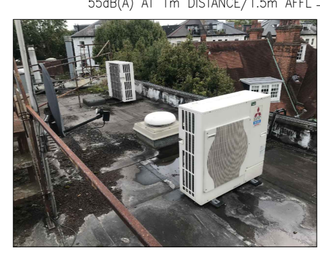
MITSUBISHI ?? CONDENSING UNIT ANTICIPATED SOUND PRESSURE LEVEL: 55dB(A) AT 1m DISTANCE/1.5m AFFL
