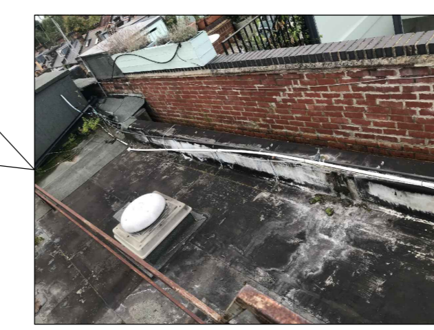
ROOF MOUNTED EXTRACT FAN ANTICIPATED SOUND PRESSURE LEVEL: 48dB(A) AT 3m DISTANCE ADJACENT PROPERTY
