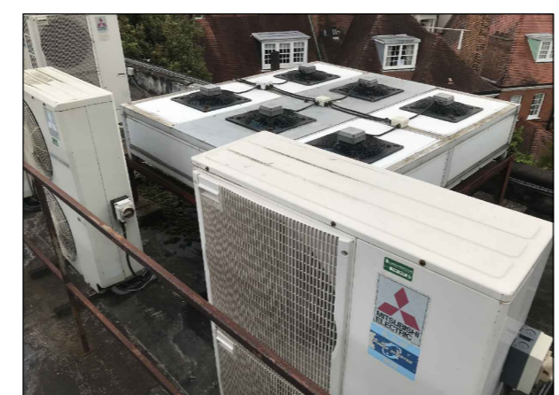
UNKNOWN DRY AIR COOLER ANTICIPATED SOUND PRESSURE LEVEL: 52dB(A) AT 1m DISTANCE/1.5m AFFL
