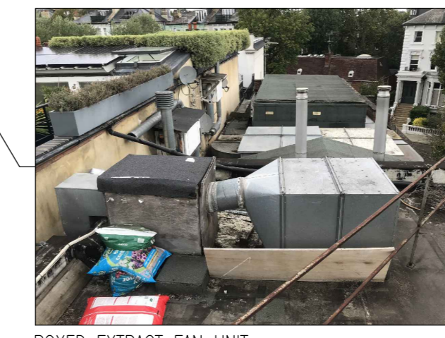
ROOFED EXTRACT FAN UNIT ANTICIPATED SOUND PRESSURE LEVEL: 55dB(A) AT 1m DISTANCE/1.5m AFFL
