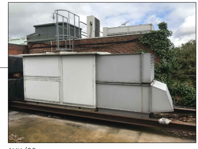
AHU/02 UNKNOWN NOISE INFORMATION, ASSUMED SIMILAR TO NEW UNIT (DETAILS OPPOSITE) BUT FACTOR IN A 10% WORSENING FOR AGE OF CONSTRUCTION AND CONDITION
