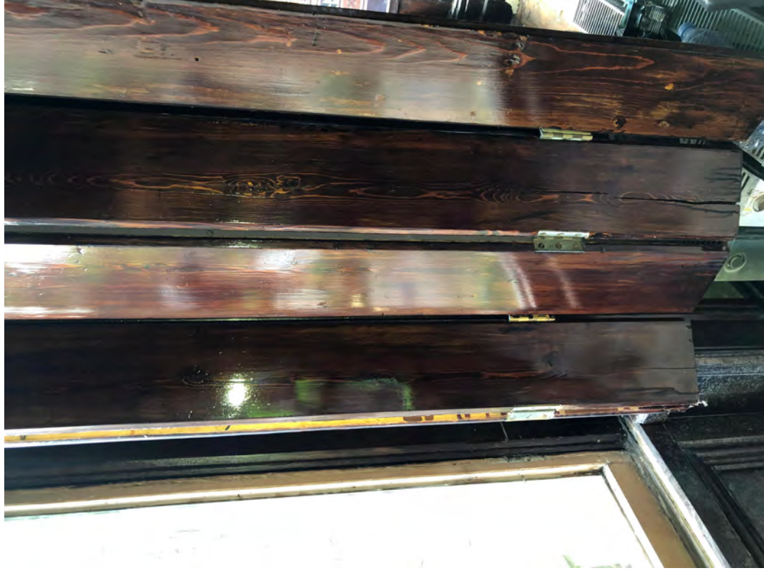
Figure 26: The timber base of the shutters is of modern softwood, thickly coated with a dark varnish to loosely imitate the original joinery
