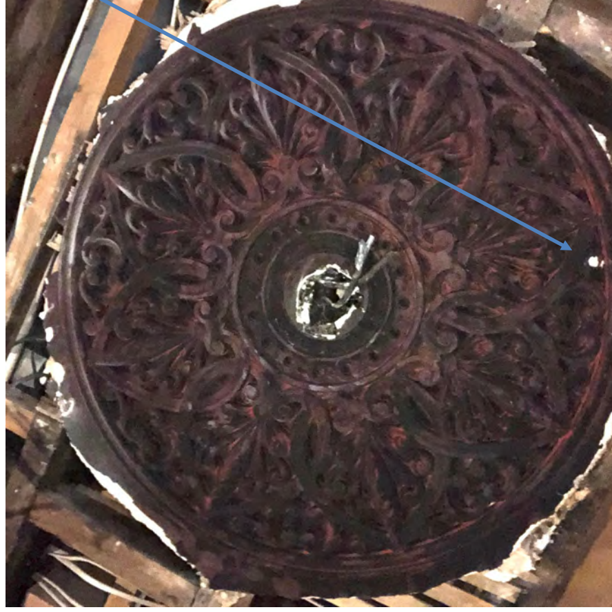
Figure 7: Room 1 Ceiling Rose
