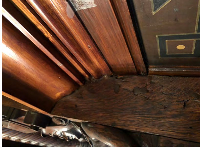
Figure 64: Room 3, mismatch of timber types and finishes. Also, poorly aligned joints, which suggests a recent reworking.
