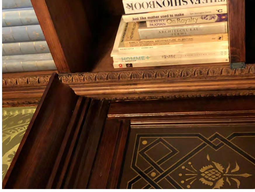
Figure 66: Jarred alignment of the modern cornice to the panels and the historic bookcase.
