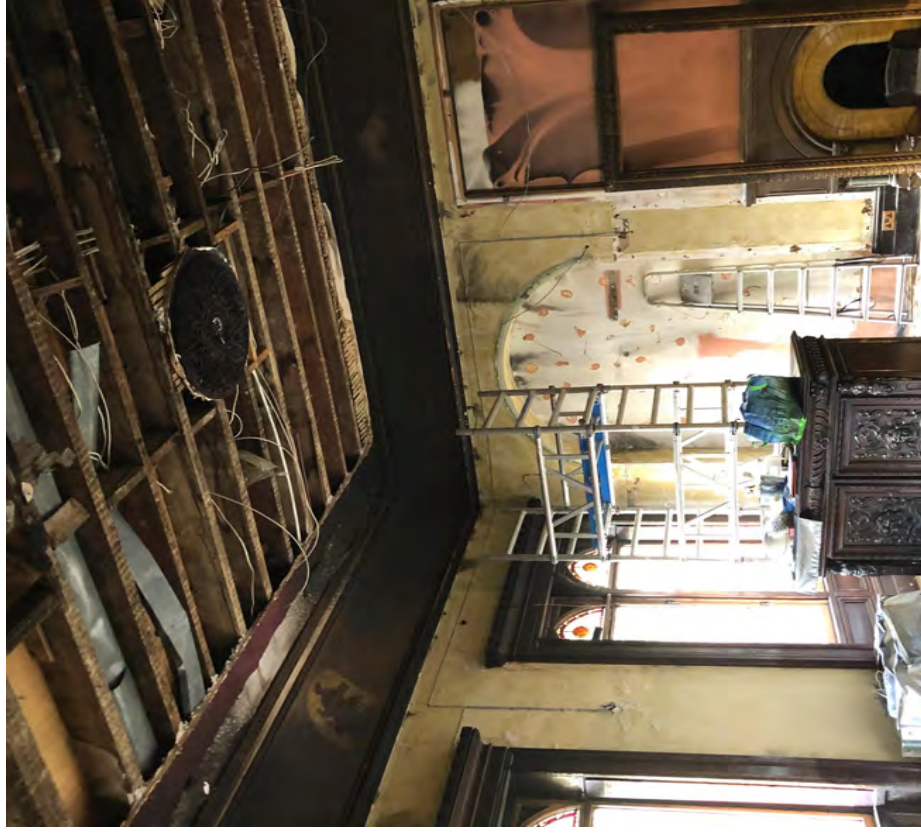
Figure 4: Room 1, Reception after the fire (approximately the same orientation)
