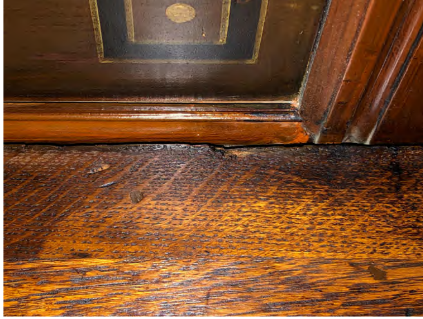
Figure 65: Room 3, poor alignment of panels and adjacent mouldings which again would suggest a more recent reworking of the interior.
