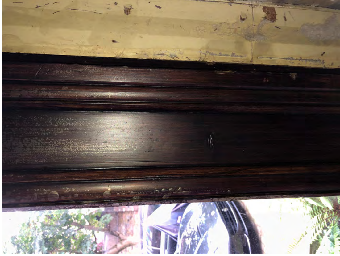
Figure 23: Window joinery showing the retouched original scheme beneath a degraded later acrylic varnish
