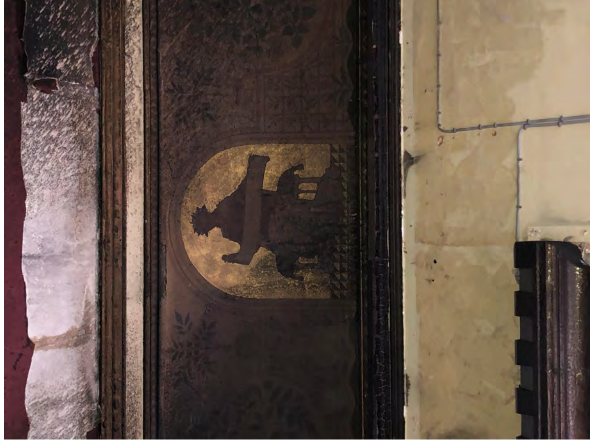
Figure 33: frieze area above the source of the fire after initial clean
