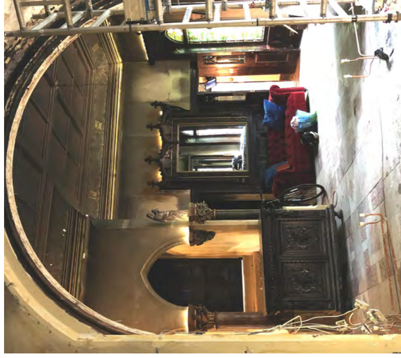
Figure 37: Room 2. Entrance Hall after the fire
