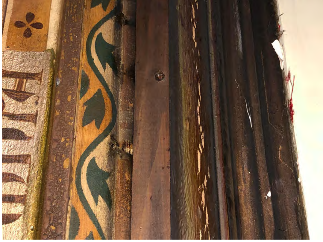
Figure 34: Detail of frieze showing bubbling to the paint layers and the buckled modern plastic conduits for recent cable installations (not included in this report)
