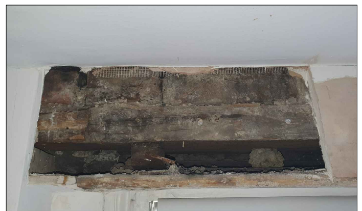
Photo taken from the 3rd floor rear bedroom. Existing timber lintel and brickwork above windows in very poor condition
