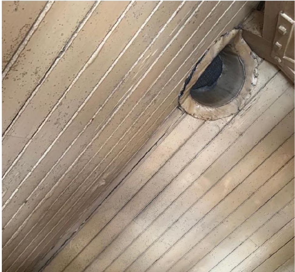
Close boarded attic ridge with the internal opening for the roof ventilation cowl. Also visible are marks caused by the mould growth on the boarded soffit due to lack of roof space ventilation
