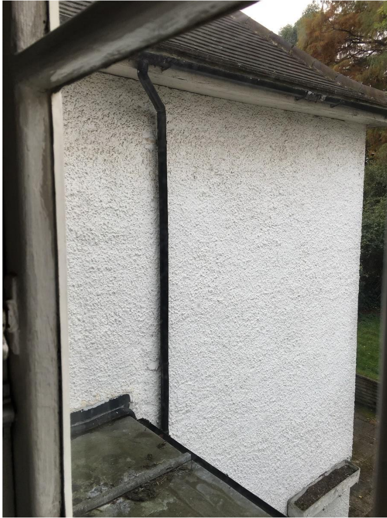
Figure 8 – Photo of the rear pebble-dashed flank wall of no.75 Lawn Road, dated October 2017. It is proposed to be demolished under this application.
