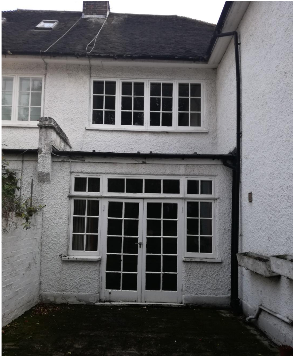
Figure 7 – Photo of the rear of no.75 Lawn Road dated October 2017. The existing first floor wall and part of the flank wall is proposed to be demolished under this application.
