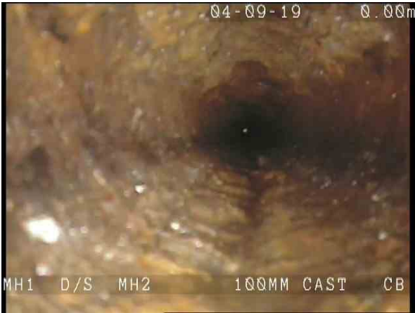
MH1X_697d6ba7-1a86-43ea-9b00-4985f68a1723_20190906_095824_558.jpg, 00:00:06, 0.10 m Attached deposits, encrustation from 12 o'clock to 12 o'clock, 5% cross-sectional area loss, start
