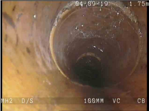
MH2X_99a95e93-e9bd-4658-b633-a5a8b0b76c35_20190906_101510_209.jpg, 00:00:33, 1.80 m Crack, circumferential at joint from 8 o'clock to 3 o'clock
