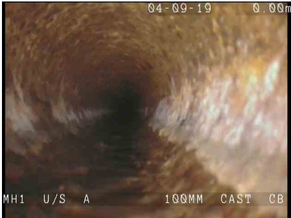
A_MH1X_7069cf84-8557-4d21-aaf6-a844871a4e0a_20190906_100331_033.jpg, 00:00:03, 0.10 m Attached deposits, encrustation from 12 o'clock to 12 o'clock, 5% cross-sectional area loss, start
