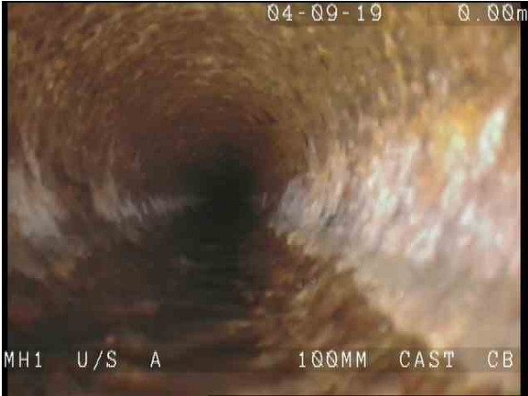
A_MH1X_7069cf84-8557-4d21-aaf6-a844871a4e0a_20190906_100331_033.jpg, 00:00:03, 0.10 m Attached deposits, encrustation from 12 o'clock to 12 o'clock, 5% cross-sectional area loss, start
