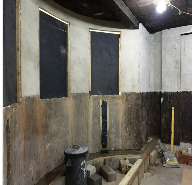
Image 6 – View of bay windows internally noting the head height is close to the soffit preventing the windows from matching the height of existing bay windows above
