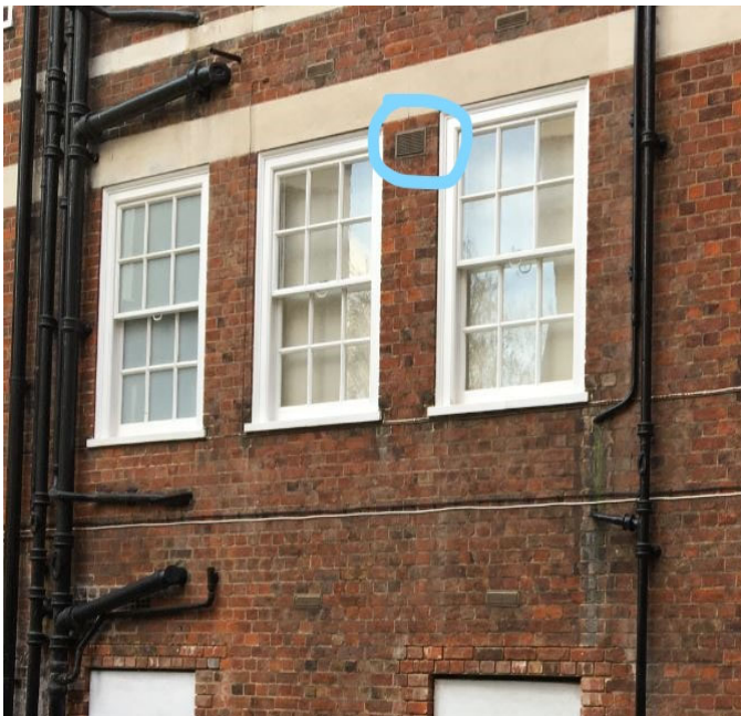
Image 3 – Example of existing extractor vent cover. New covers to be brown to match.
