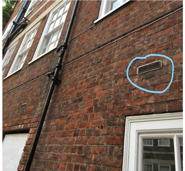
Image 2 – Example of existing airbrick cover in plastic and metal.
