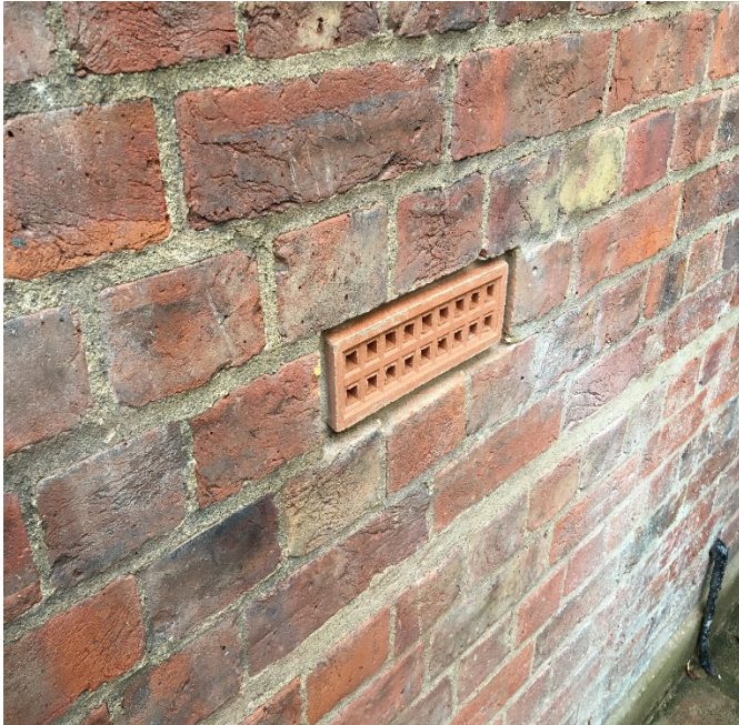
Image 1 – Terracotta airbricks installed to underfloor vents in lieu of plastic and metal
