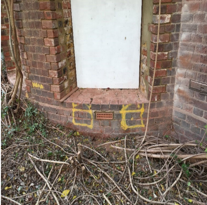
Image 5 – View of bay windows externally noting the cill height is at dpc and ground level restricting a match of the height of existing bay windows above.
