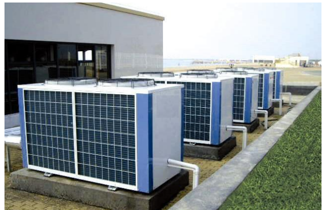
Figure 6: Outdoor units of ASHP
