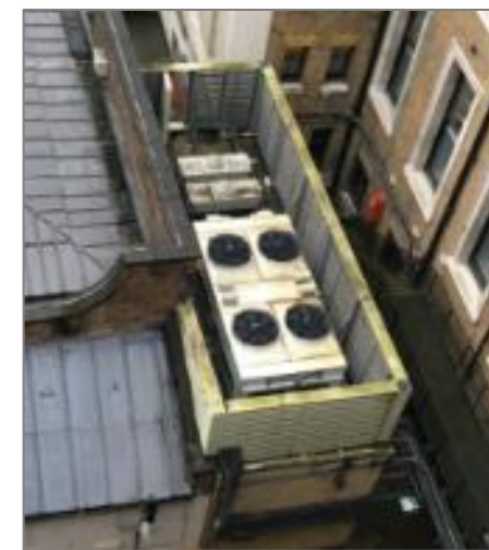
Figure 2—3 Existing Gallery 1 condenser within the plant compound
