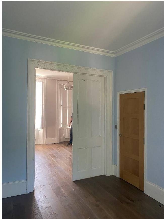
A photograph of one of the existing modern doors next to the traditional panelled doors between bedroom F02.0 and F03.0.
