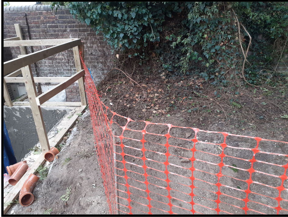
Photo 3: Proximity of basement to tree T01
