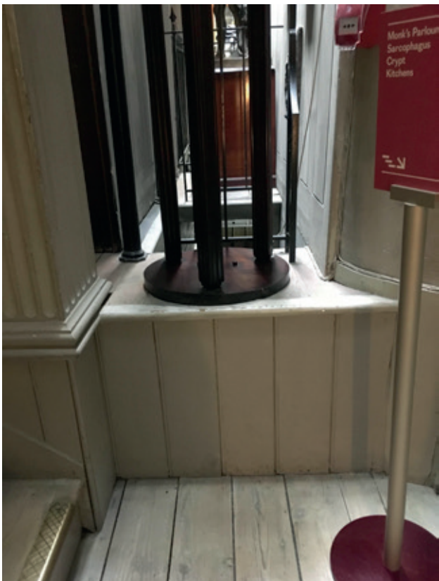
Figure 29 (Top Left): Area to the west of the half landing on the Basement Stairs (top), 2019. Figure 31 (Top Left): Area to the west of the half landing on the Basement Stairs (bottom), 2019.
