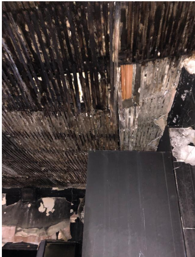
Photo 29 - sagging trimmer joist at second floor level above Apartment 9
