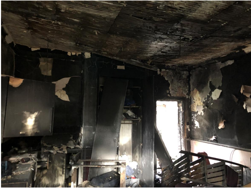
Photo 28 - sagging trimmer joist at second floor level above Apartment 9
