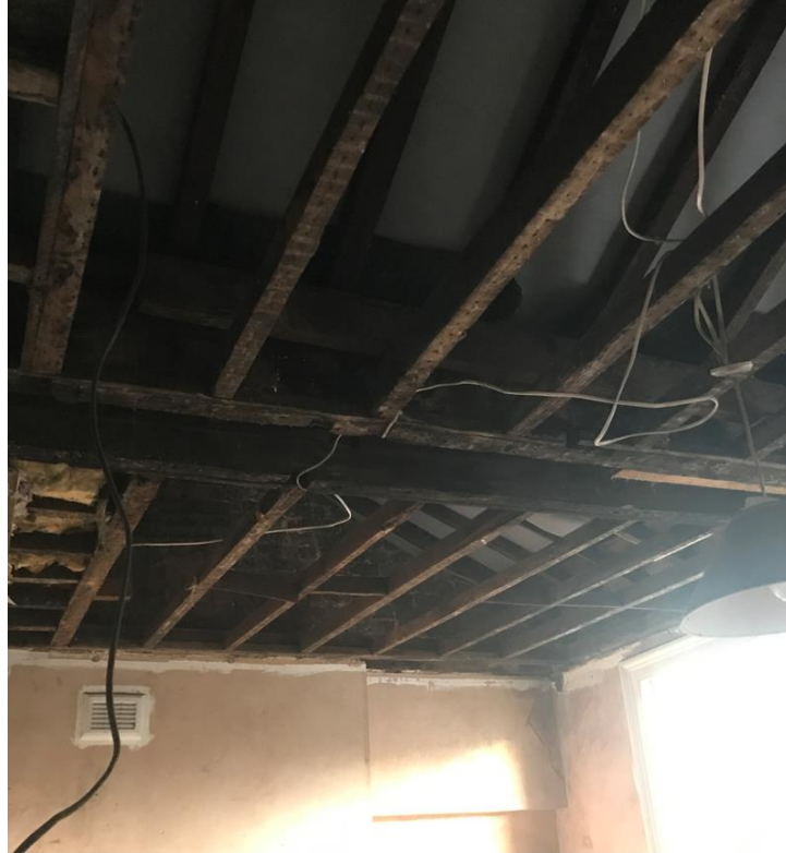
Fig. 9 Photo of rafters taken by client prior to the consented removal of the butterfly roof.
