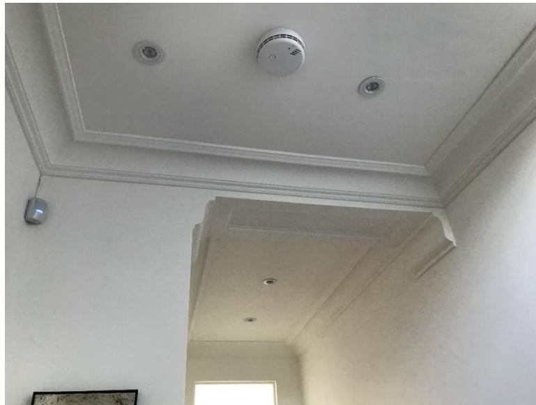
Fig. 10 Spotlights to the entrance hall and main stair area
