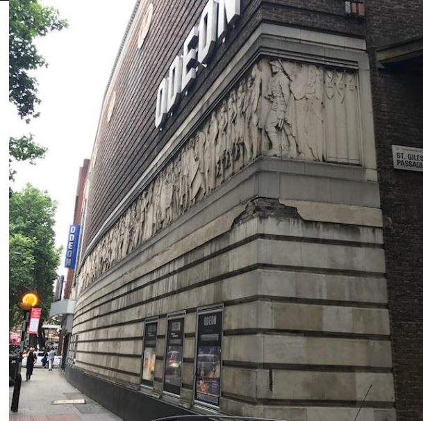
Damage to stonework of frieze
