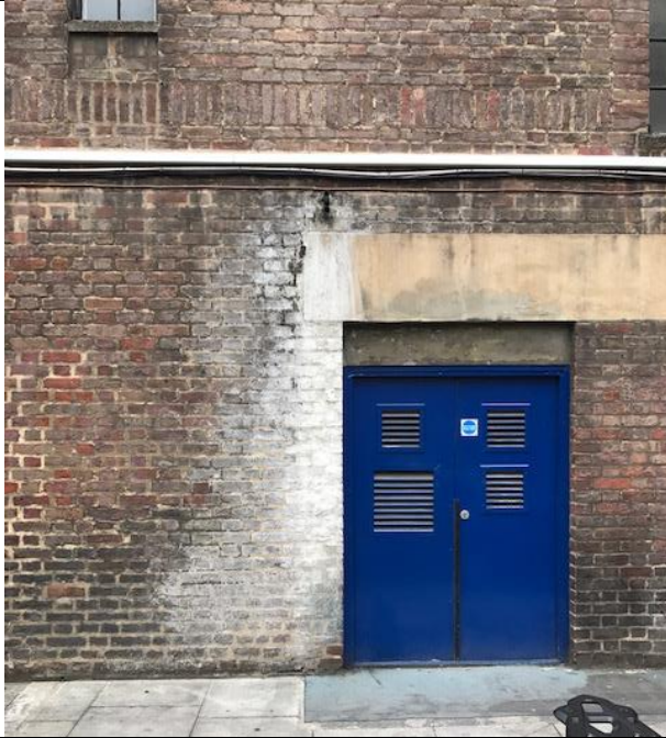
Damage caused to brickwork of rear elevation by defective overflow.
