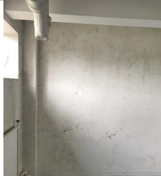
Wall to unused office affected by penetrating dampness
