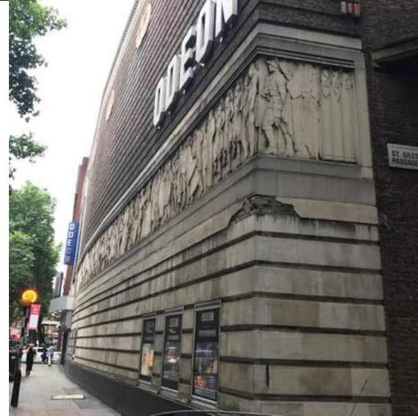
Damage to stonework of frieze
