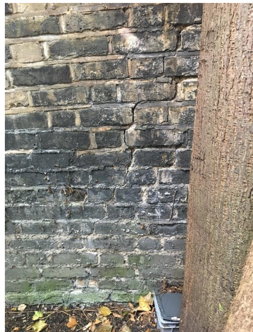
Figure 4: T5 Lime close to boundary wall with stepped cracking.
