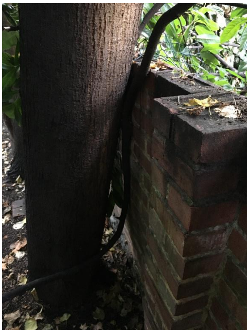
Figure 3: T4 Lime leaning on rear boundary wall.
