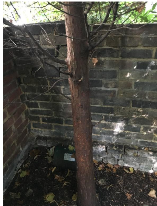
Figure 2: T3 Cypress close to boundary wall with cracking.
