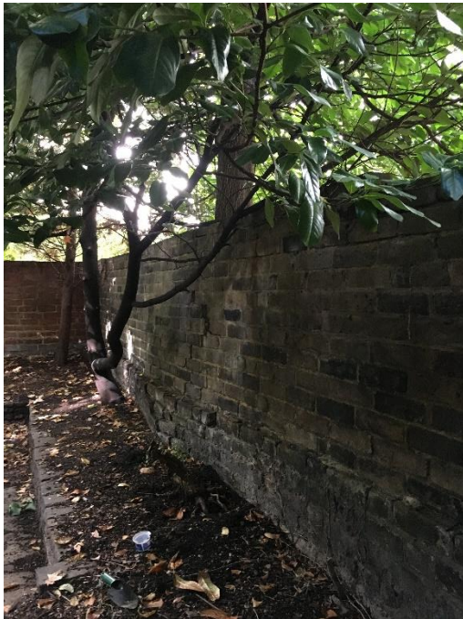
Figure 1: T1 and bulging boundary wall.
