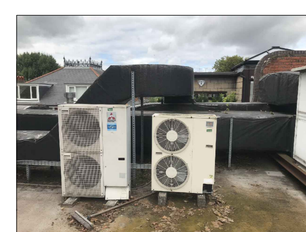
LEFT: MITSUBISHI PUH2-RP5YHA CONDENSING UNIT ANTICIPATED SOUND PRESSURE LEVEL: 52dB(A) AT 1m DISTANCE/1.5m AFFL RIGHT: HITACHI RAS-4HQVES CONDENSING UNIT ANTICIPATED SOUND PRESSURE LEVEL: 49dB(A) AT 1m DISTANCE/1.5m AFFL
