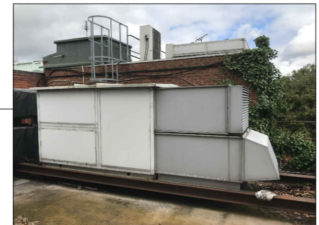
AHU/02 UNKNOWN NOISE INFORMATION, ASSUMED SIMILAR TO NEW UNIT (DETAILS OPPOSITE) BUT FACTOR IN A 10% WORSENING FOR AGE OF CONSTRUCTION AND CONDITION
