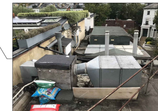
ROOF MOUNTED EXTRACT FAN ANTICIPATED SOUND PRESSURE LEVEL: 48dB(A) AT 3m DISTANCE ADJACENT PROPERTY
