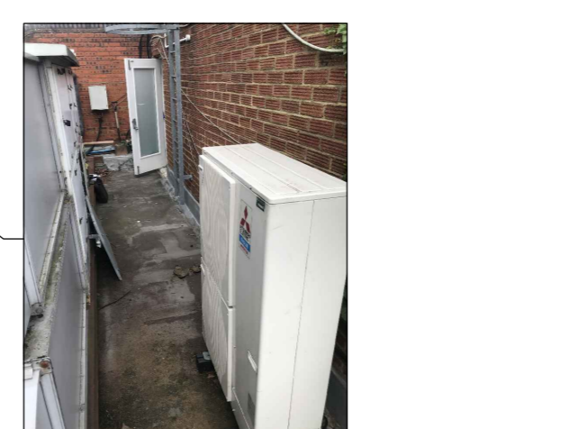
MITSUBISHI ?? CONDENSING UNIT ANTICIPATED SOUND PRESSURE LEVEL: 55dB(A) AT 1m DISTANCE/1.5m AFFL
