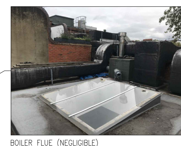
BOILER FLUE (NFGUGBL1)
