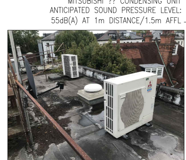
MITSUBISHI ?? CONDENSING UNIT ANTICIPATED SOUND PRESSURE LEVEL: 55dB(A) AT 1m DISTANCE/1.5m AFFL
