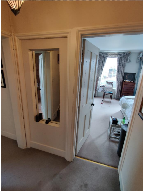
The landing outside the first floor Master Bedroom. Note the infilled doorway on the left, evidence of a previous undetermined room or landing layout.
