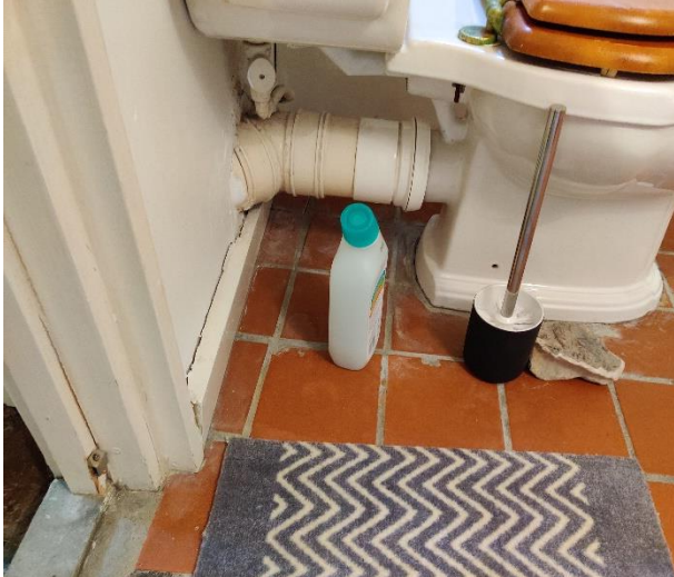
Close-up of above-ground soil pipe. The new connection would be above ground, on the side of the pipe closest the WC window.
