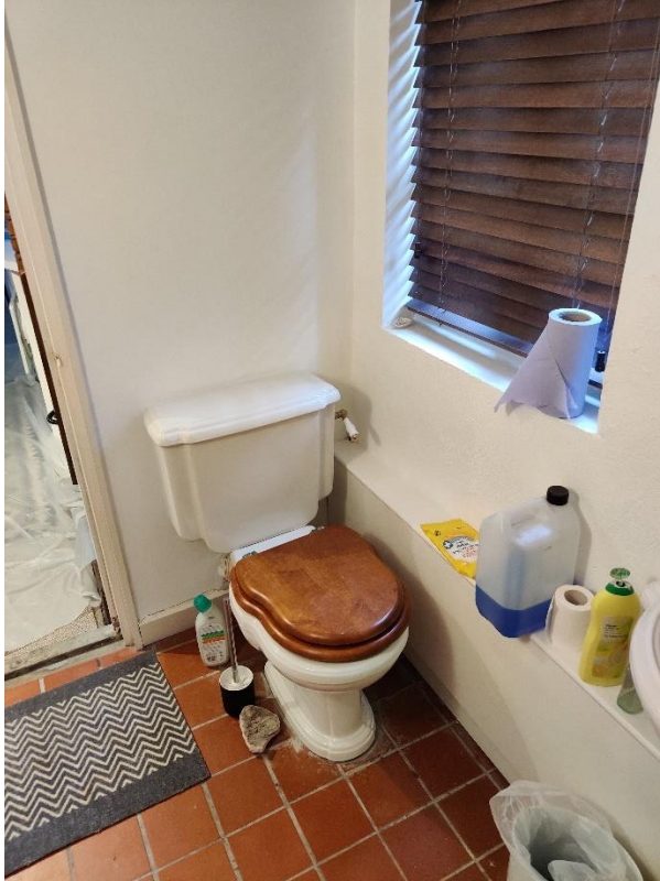
The cellar WC. All finishes and sanitaryware are C20 and by the previous owner. Note the pipework boxing concealing the supply and waste pipework to the sink (right-hand-side, out of shot).
