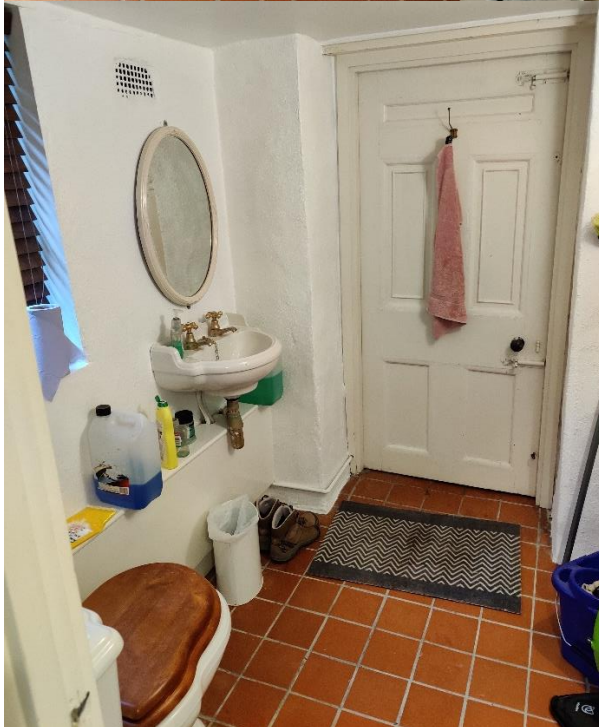
The cellar WC. The new pipework would be inserted in the corner just to the right of the mirror, and would return along the existing pipework run.
