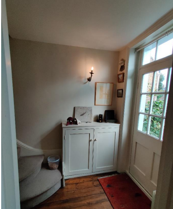
The ground level entrance hall, with C20 built-in cabinet to be replaced
