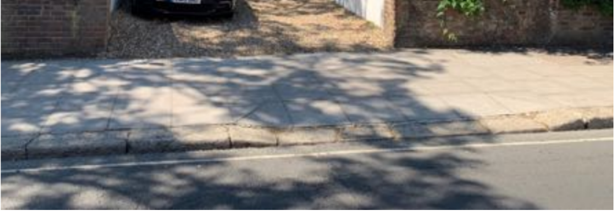
3: Misalignment of the crossover
