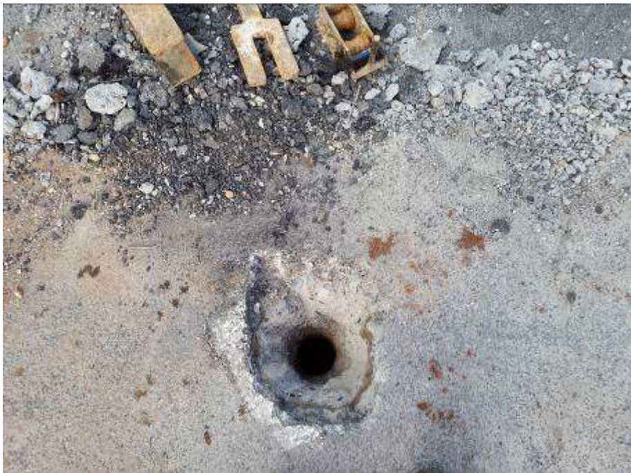
Plate 4 Showing concrete below blacktop
