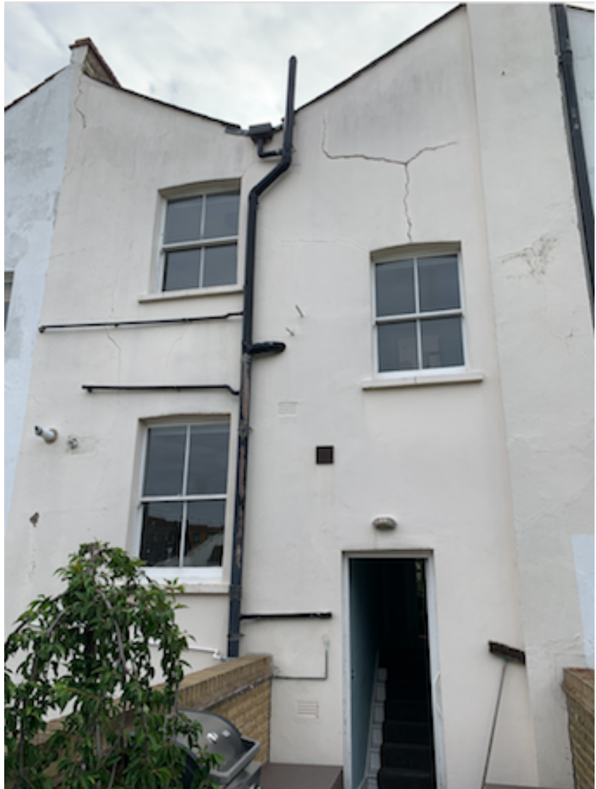
View of rear elevation of 41 Leverton Street taken from the first-floor terrace
