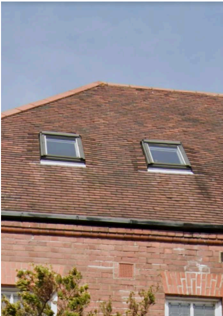
Existing Materiality, showing the conservation windows already installed in the front elevation
