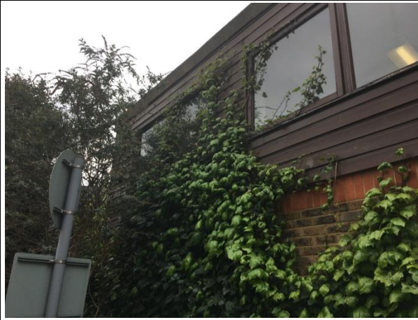
Photo 2. Ivy growing on south eastern corner of Jules Thorn Day Centre (B1).
