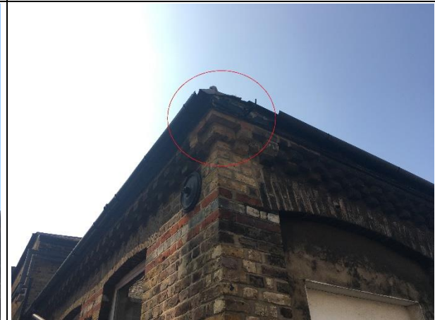
Photo 18. Broken wooden boarding on corner of the Kitchen Block (B6).
