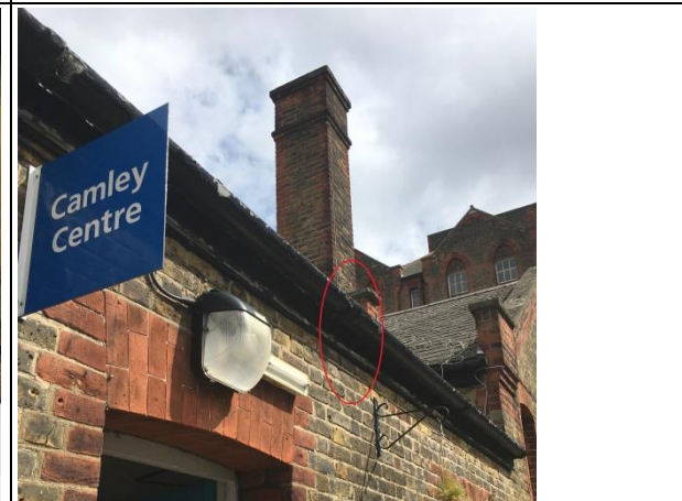
Photo 6. Gap in fascia at Camley Centre (B2).
