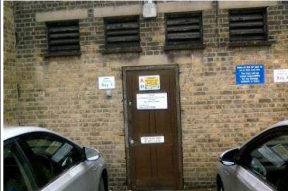
Photo 14. Switch room in the Post Room and Former Mortuary building (B5).
