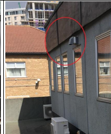
Photo 12. Gaps under the soffit at the northern elevation of the Bloomsbury Day Centre (B4).
