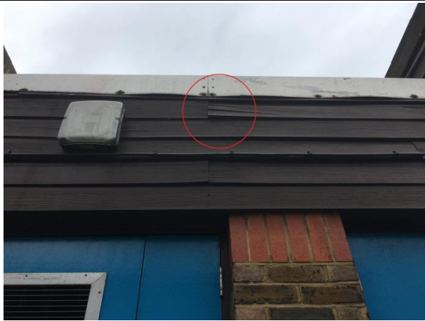
Photo 1. Gap under wooden cladding on southern elevation of Jules Thorn Day Centre (B1).
