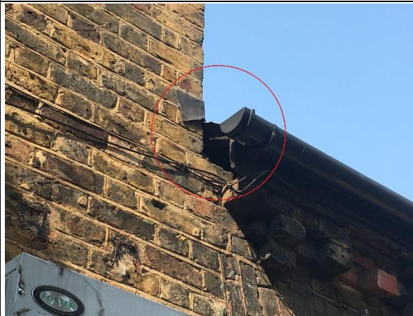
Photo 17. Gap in wooden boarding (beside security light) on the Kitchen Block (B6).
