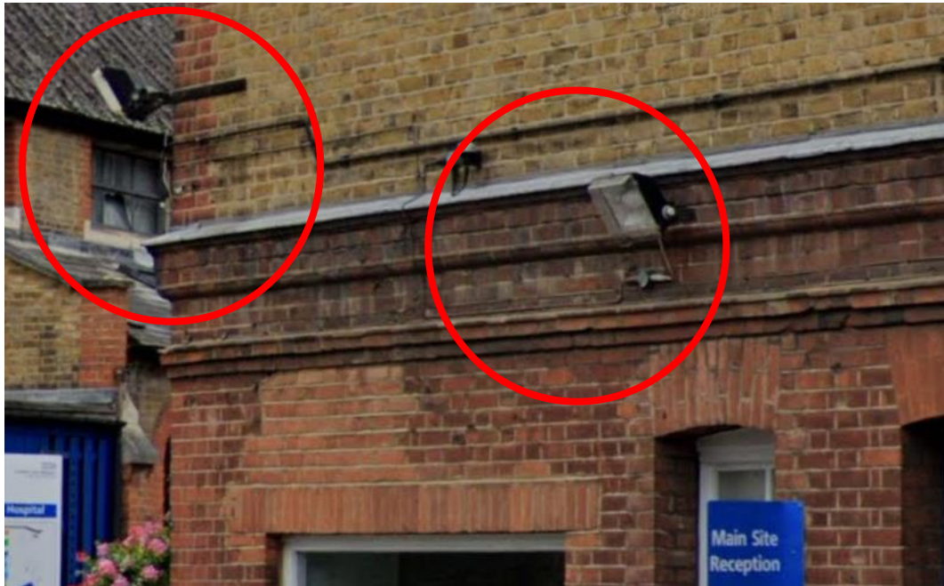
Figure 4-6 Existing Site Entrance Wall Lighting
