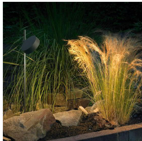
Lighting inside planters
