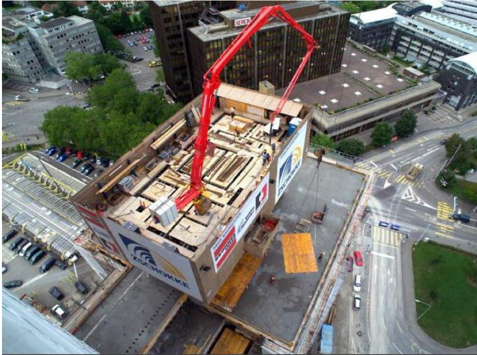
Figure 3-5: Indicative only - Ariel View of a Doka SCP 400 showing upper storage platform in use
