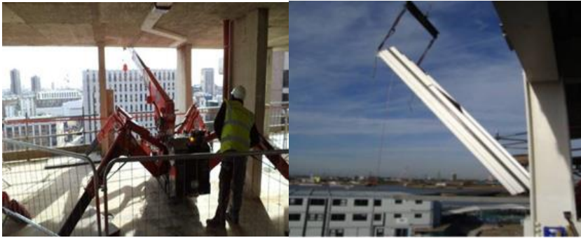
Figure 3-6: Example of spider crane from the floor above lifting panel into place
