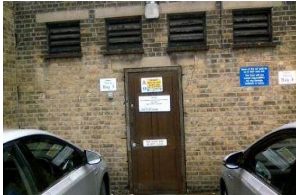
Photo 14. Switch room in the Mortuary building (B5).
