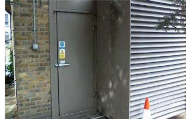
Photo 15. Generator room in the Mortuary building (B5).
