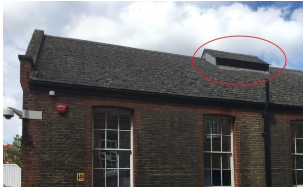
Photo 8. Elevated roof vent on the Camley Centre (B2).
