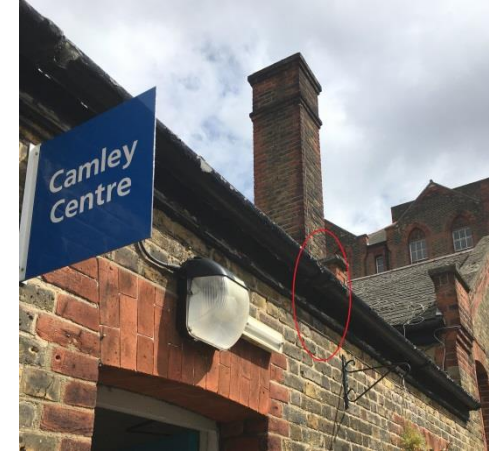
Photo 6. Gap in fascia at Camley Centre (B2).
