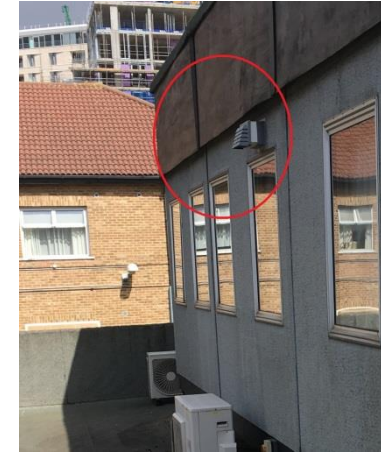
Photo 12. Gaps under the soffit at the northern elevation of the Bloomsbury Building (B4).
