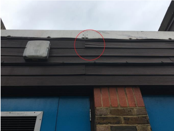
Photo 1. Gap under wooden cladding on southern elevation of Jules Thorn (B1).
