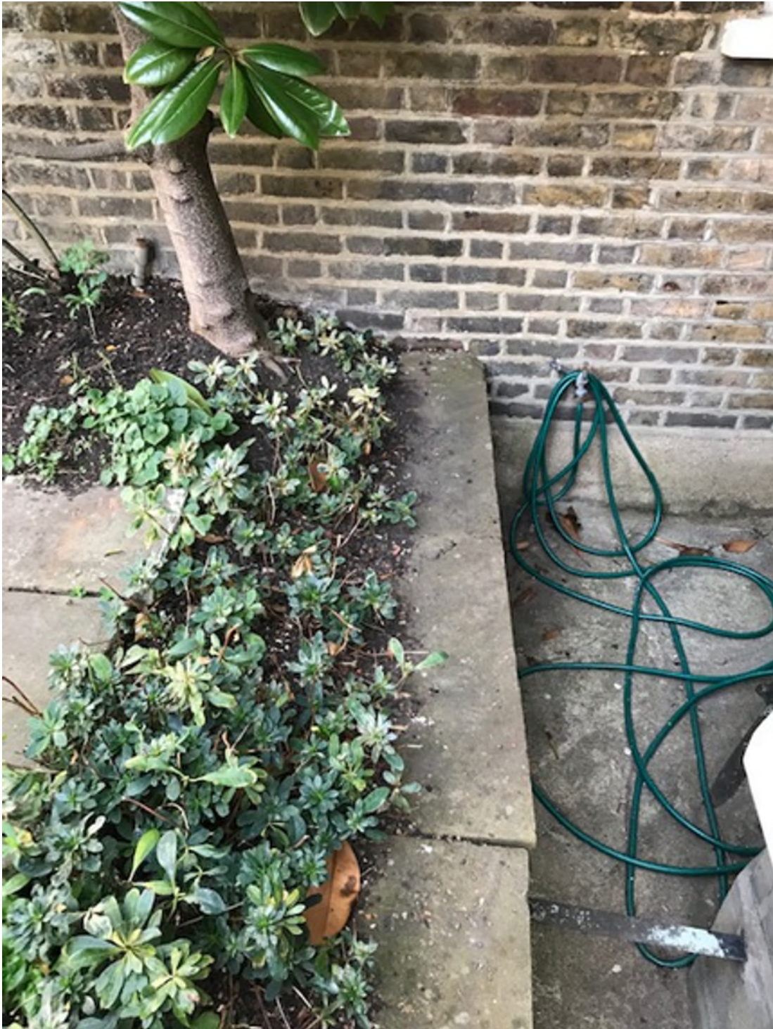
Photograph 2 – Showing proximity to wall and dislodging of capping stone.
