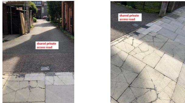
Figure 1.8 - Damage to pavement entrance to shared private road
