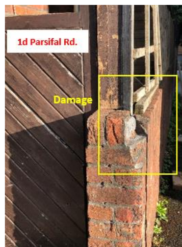
Figure 1.5 - Damage to boundary wall of 1d Parsifal Rd. by previous reversing vehicles
