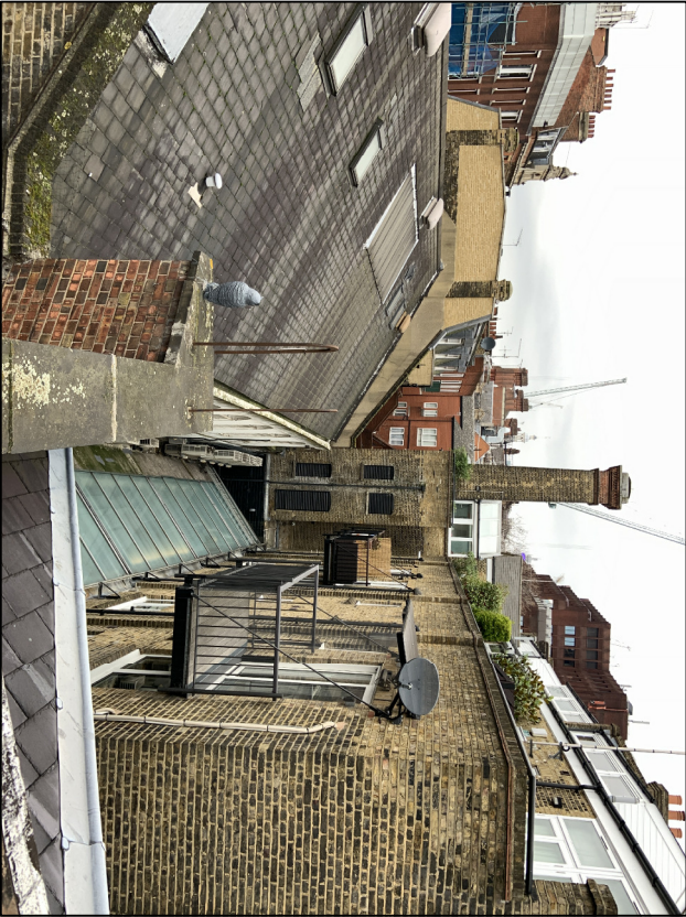
2No existing MVHR Roof Cows to be retained
