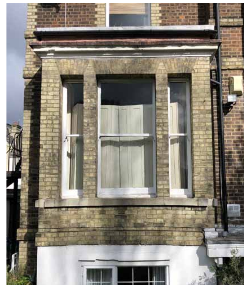
s) Rear secondary bay showing subsidence of both sides.
