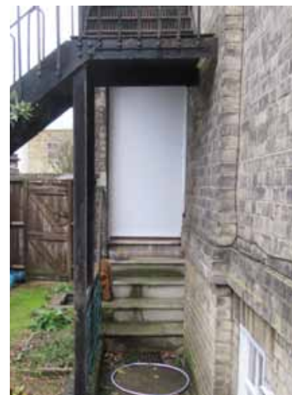
n) View of existing rear door and entrance steps to be removed.
