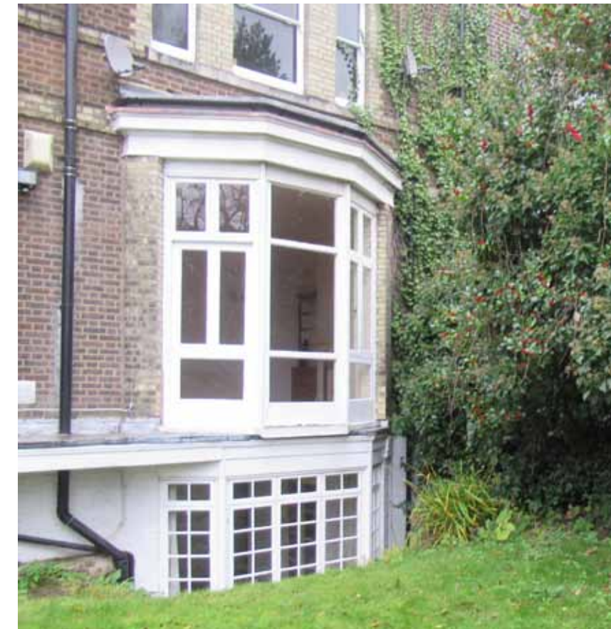
p) View of existing re-built main rear bay, redundant platform, un-orderly soil pipes and satellite dishes
