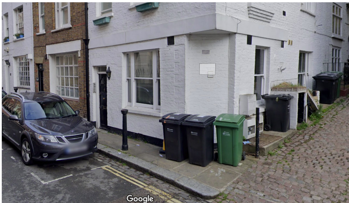
Nos. 13 and 15 – Concrete lintels in replacement of original shopfront bressumers? Note disturbed brickwork on front façade adjoining cut corner at ground floor level (original shopfront entrance?)
