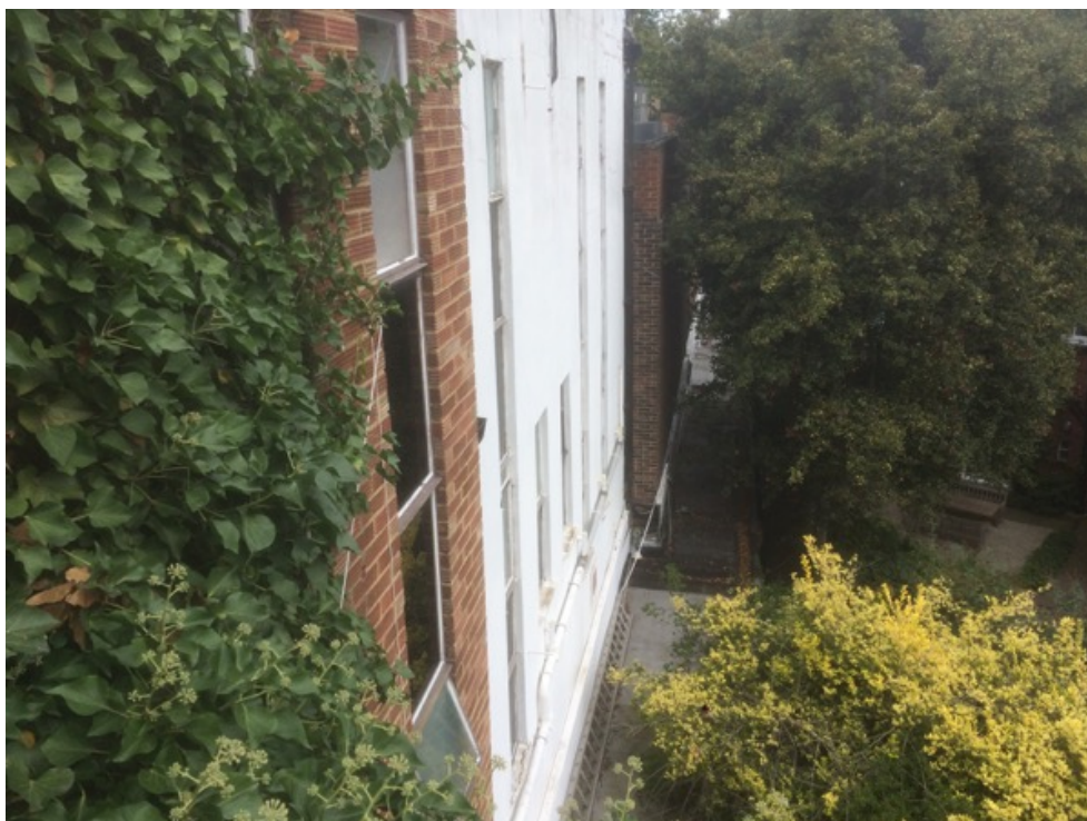
Fig 17: No. 81 Belsize Park Gardens – View of south east elevation facing private gardens.
