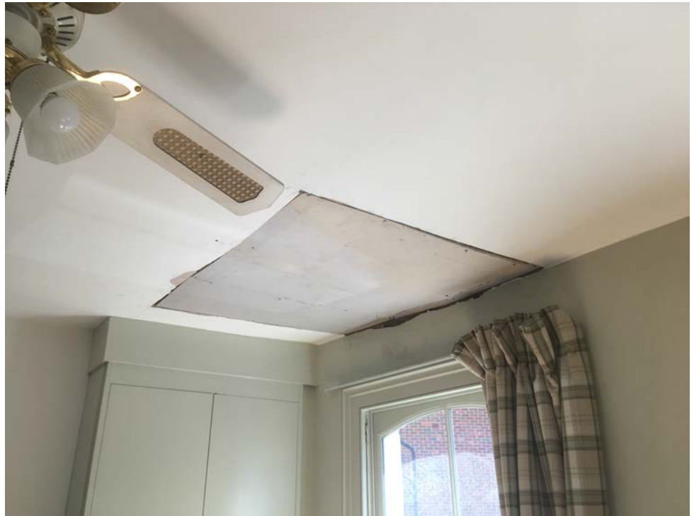
Internal damage due to water ingress
