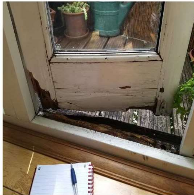
Photograph 06 – Timber Balcony doors in disrepair
