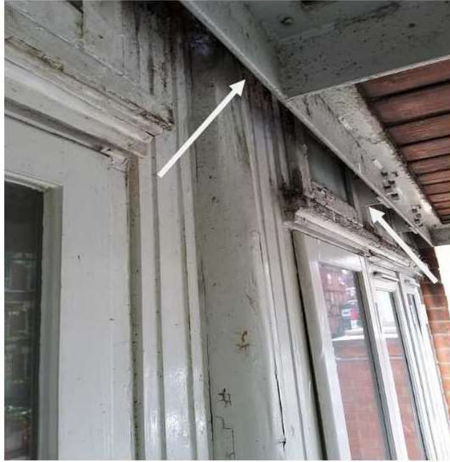
Photograph 07 – Timber Balcony doors in disrepair
