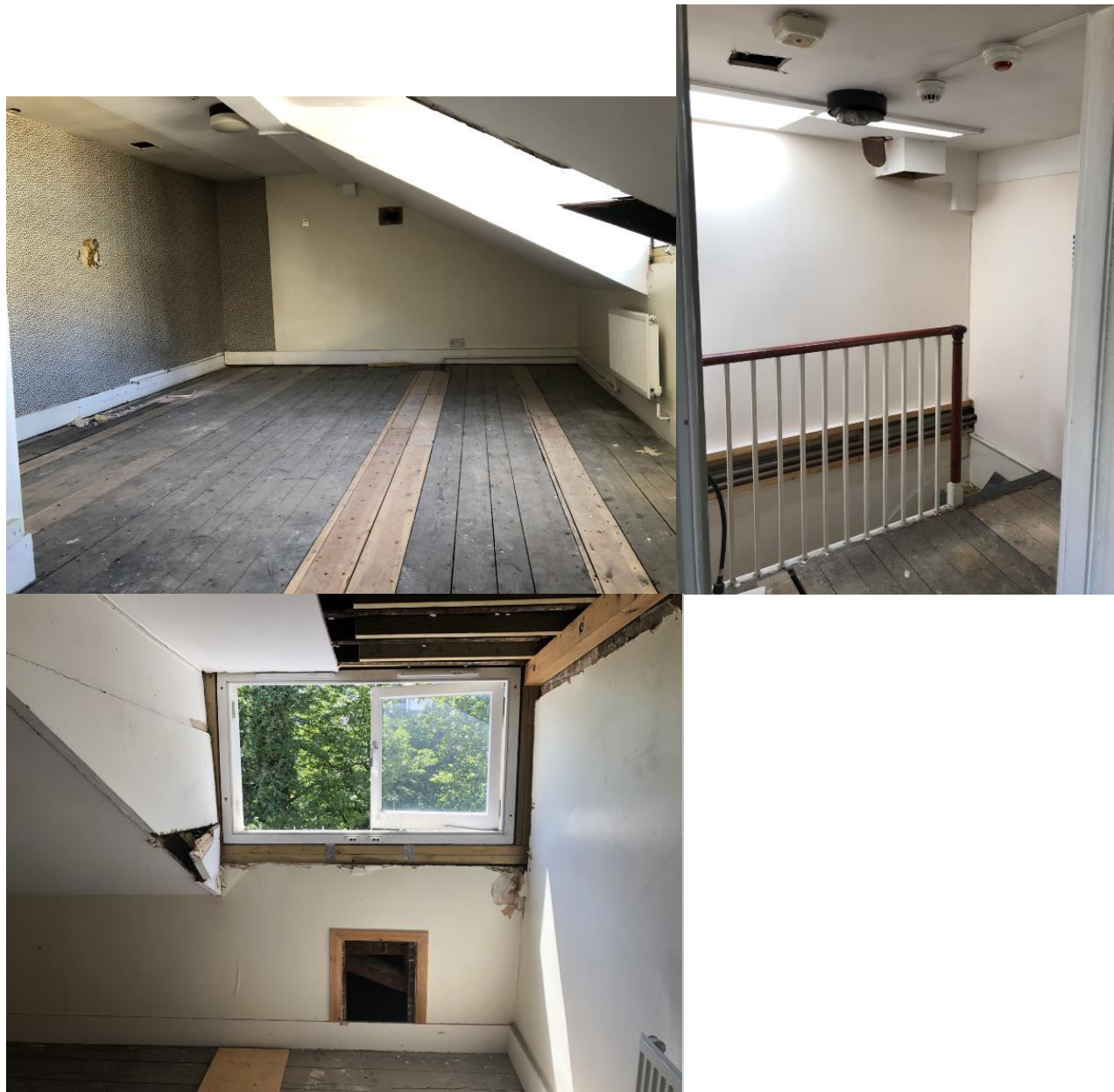
Figure 16: Photographs of fourth floor. Top: front room, landing. Bottom: rear modern window. (Source: Author's own)
