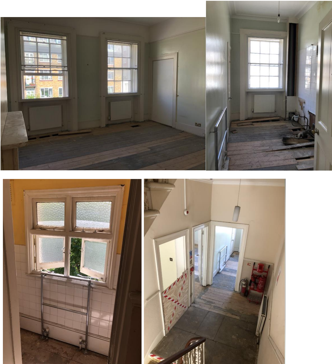
Figure 14: Photographs of second floor. Clockwise starting at top left: front room showing modern doorway, existing en-suite which adjoins the front room, second floor landing, and half landing bathroom. (Source: Author's own)
