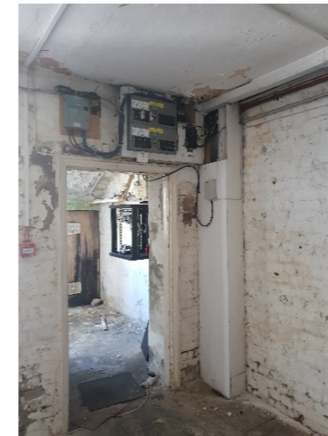
Mains Services entry in basement
