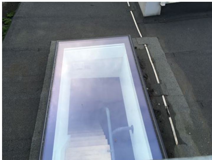
Access Roof Light at No. 9; The Proposed New Roof Light for No. 10 to Be Similar
