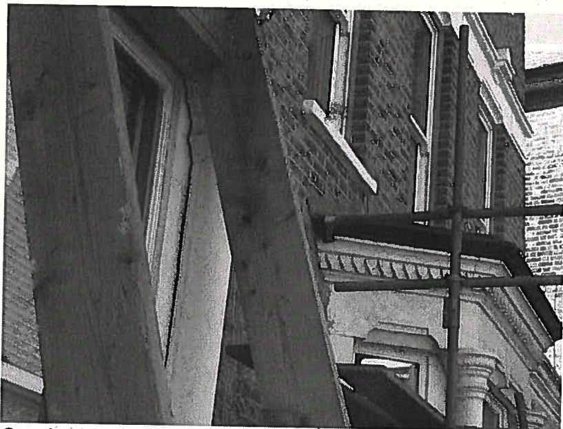
Cracked window frame and emergency structural support at 92 South Hill Park, caused by basement development next door
