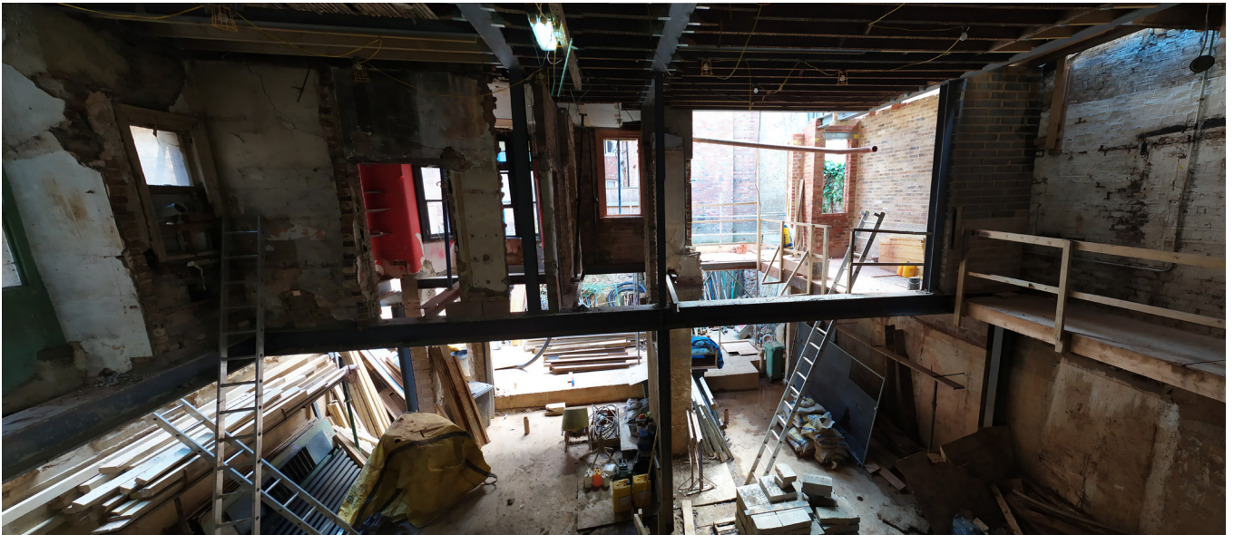
3. Rear excavated basement viewed from ground floor, retained walls and facade supported by steel beams
