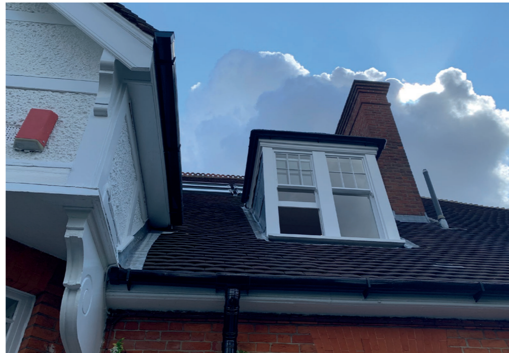
Below, The west facing roof for the proposed rooflight and the respective dormer
