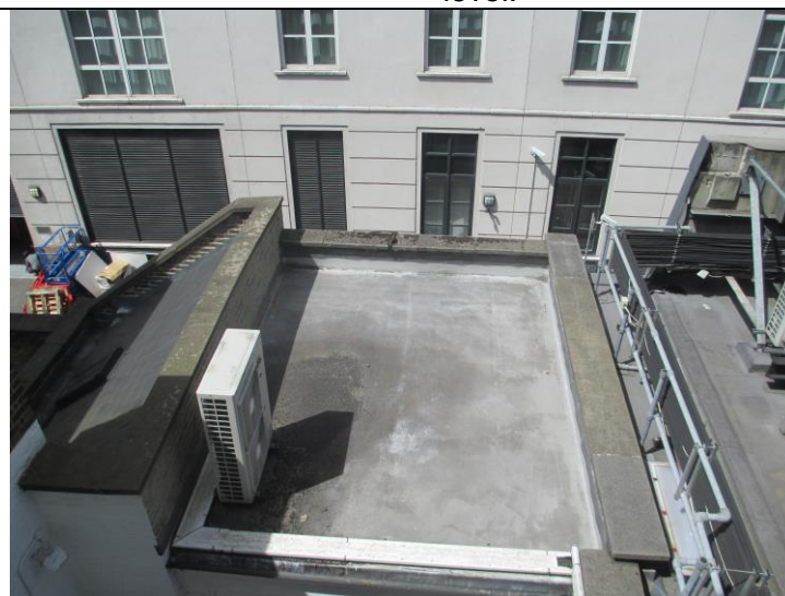
2. Roof to 2 storey rear addition where the 2 new condensers will be located.
