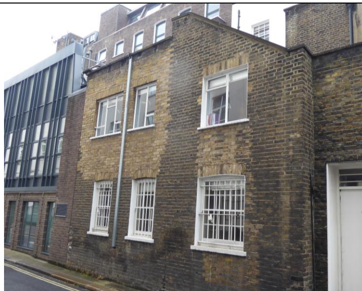
1. View of 2 storey rear addition. AC condenser will not be visible from ground level.
