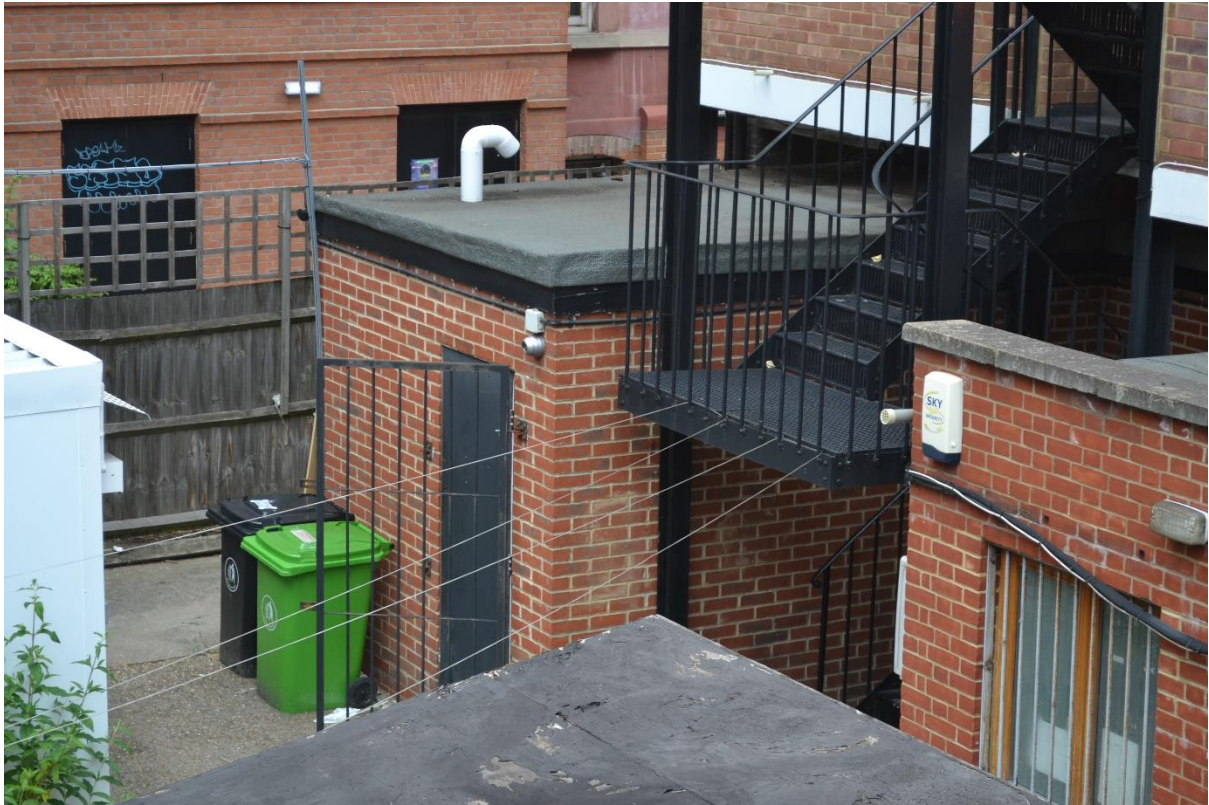
Adjoining Extension to 211 Haverstock Hill developed by the Applicant in 2007 under Planning Reference No : 2007/0784/P
