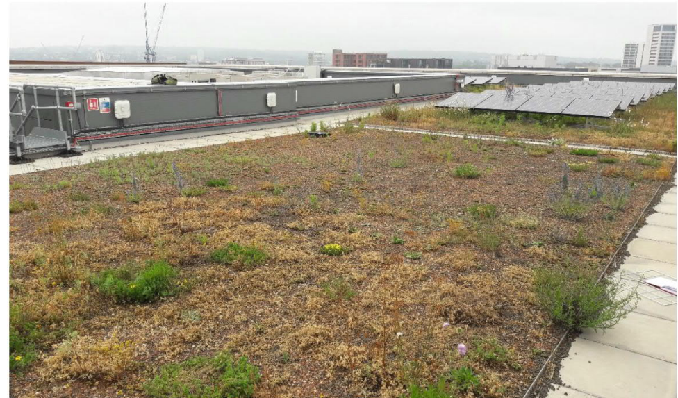
Sandy Heath Roof System at Kings Cross (~2 years) Kings Cross B6 (3 Pancras Square)
