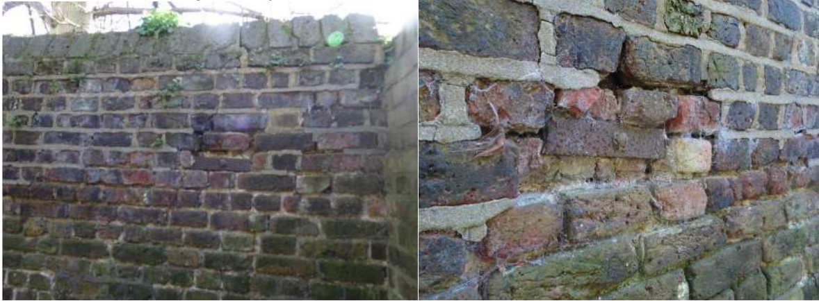
1) Boundary wall with cracking and missing mortar, varied bonding and pitted brickwork
