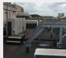
Mechanical and ventilation systems.
