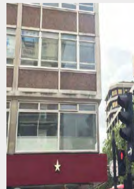
Poor thermal performance of facades and cladding.
