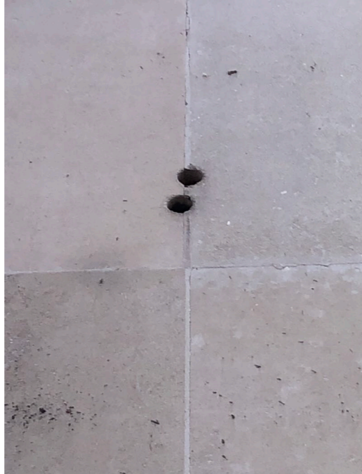
Photograph 4.7: Exterior of B4 (3 Bayley Street), mortar gaps on eastern aspect
