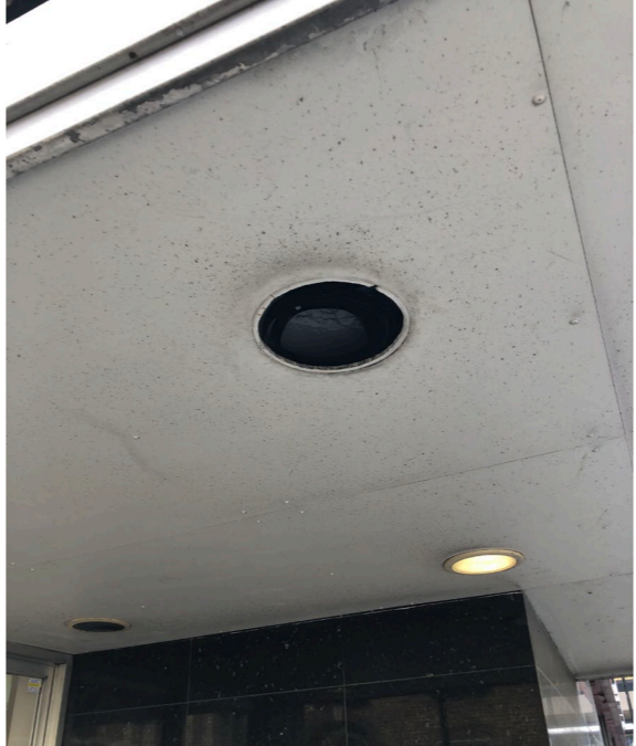
Photograph 4.8: Exterior of B4 (3 Bayley Street), missing light fitting on eastern aspect
