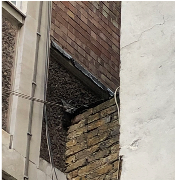
Photograph 4.4: Exterior of B2 (2 Morwell Street), gap under roof felt on southern aspect
