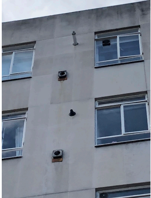
Photograph 4.6: Exterior of B4 (3 Bayley Street), mortar gap around extractor fan, eastern aspect
