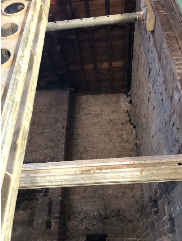
Figure 5. Detail of the crack at the corner between 165 and 163 Sumatra Road.
